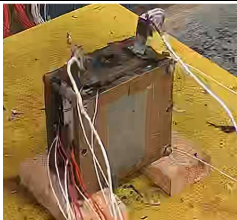
Figure 12: After thermal runaway-1
